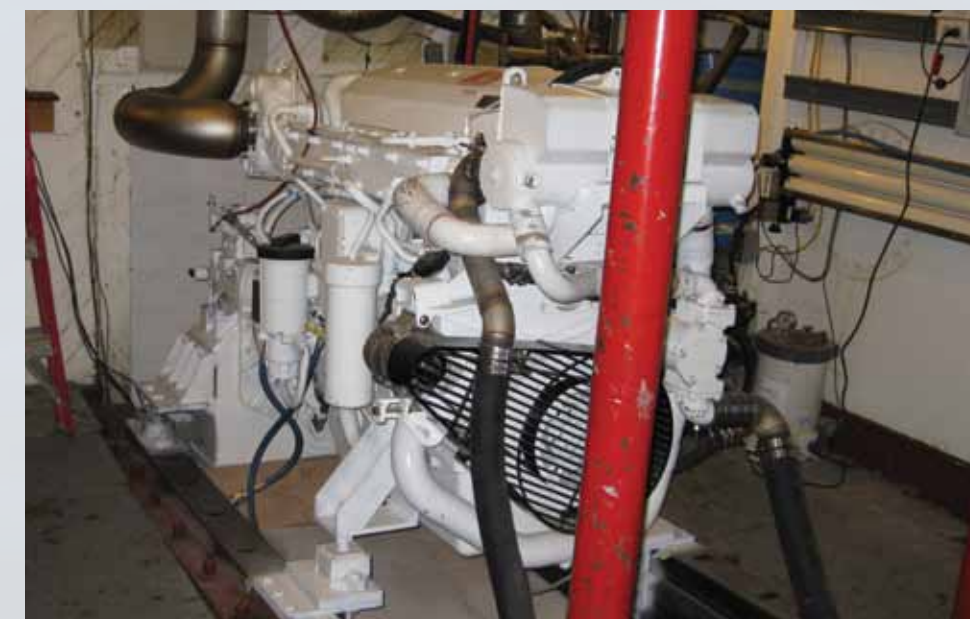
The Discovery Engine Room, After the Repower.
